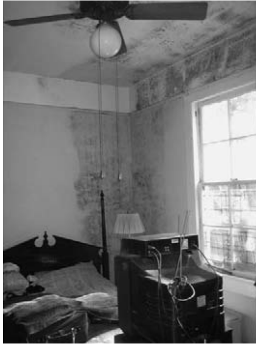
FIGURE 19.4 Mold-Damaged Building in New Orleans Following Hurricane Katrina
