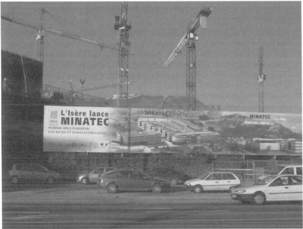
Plate 3.1 High-technology growth poles: a micro- and nanotechnology centre under construction in Grenoble, France
